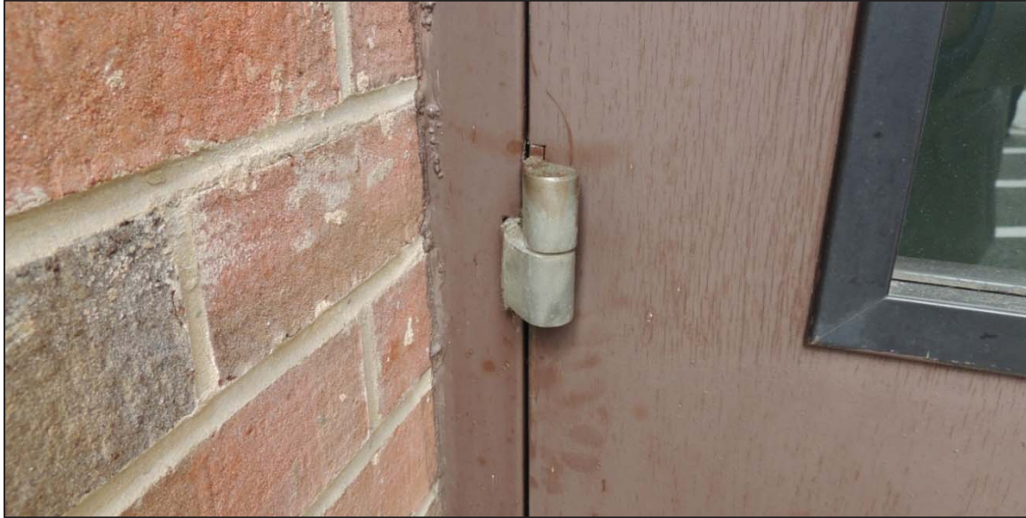
Figure 18: Exterior door with protective hinge covering.
